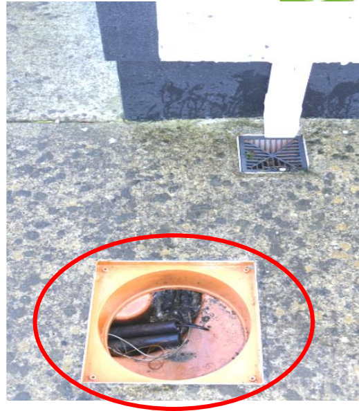
Premises where access box is fitted and duct enters premises under the floor.
