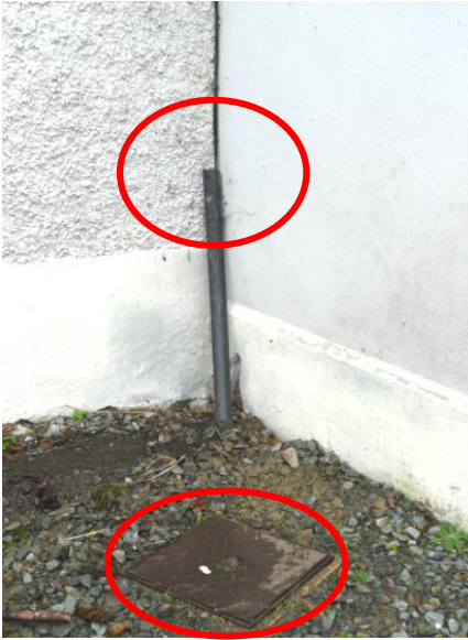
Premises where access box is fitted and duct is fitted on external wall.
